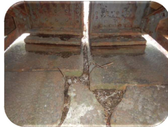
Corrosion and no evidence of 'sliding' as would be expected
