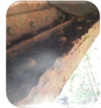
Pitting and corrosion on flanges
