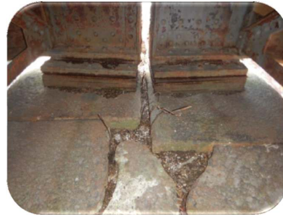
Corrosion and no evidence of 'sliding' as would be expected
