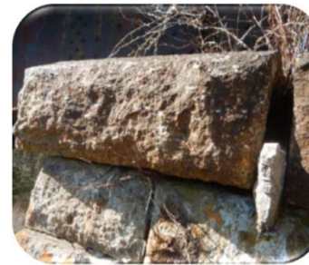
Shifting and cracked top caps – allows water to get in
