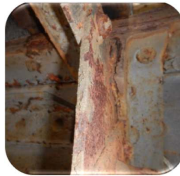
Pack rust on lateral braces
